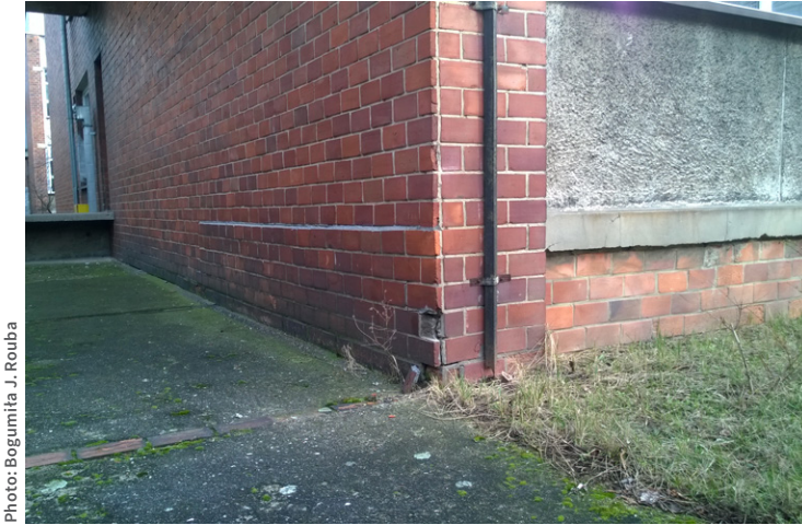
Fig. 10. This building illustrates the destructive effect of splash water bouncing from a hard concrete surface. The clinker cladding of the wall is deteriorated and detached. The other elevation, with a lawn adjacent to it, is in excellent condition.
