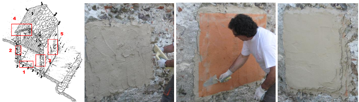
Figure 3. On the left a general view of insulations; technical phases of a thermal lime plaster
