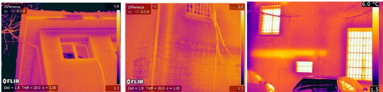
Figure 3. IR thermography investigation pre-refurbishment condition: detection of moisture in the exterior wall, rear side (left and centre); post-refurbishment IR investigation of thermal bridges: concrete stairs landing (right)
